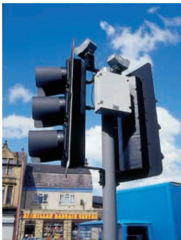
PUFFIN crossings give longer crossing times when needed and are used at many locations in West Yorkshire.
